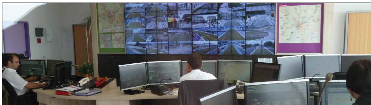
Figur 11 Kontrolcenter for letbane
